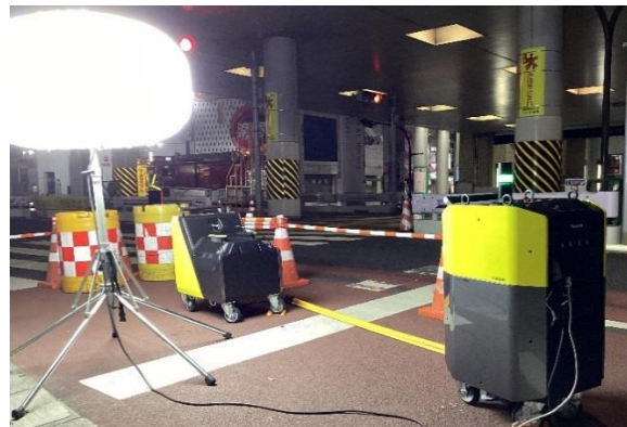
Hydrogen fuel cell generator in use as power source
